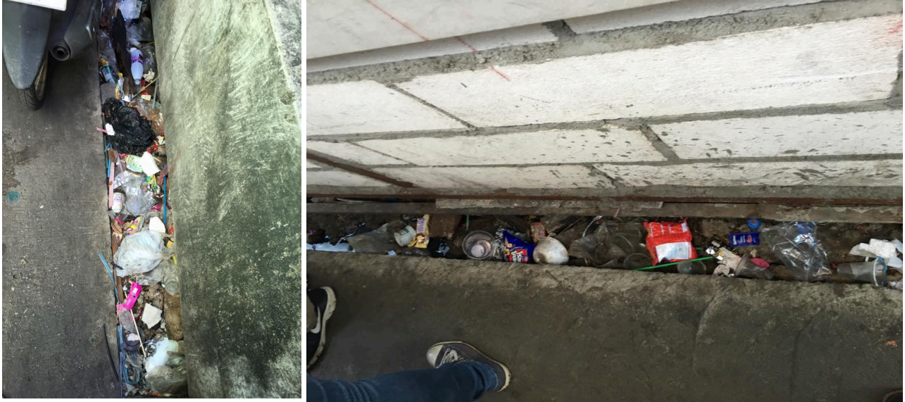
Figure 4.2 and Figure 4.3: Trash in the drainage system
