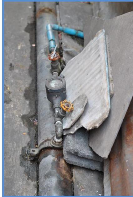
Figure 2- 4: Water Meter in the Khlong Toei Slum
