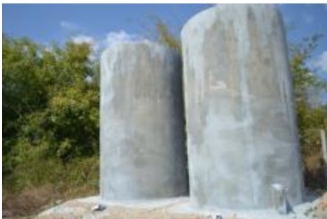
Figure 12: Water storage tank at Cabbages and Condoms
