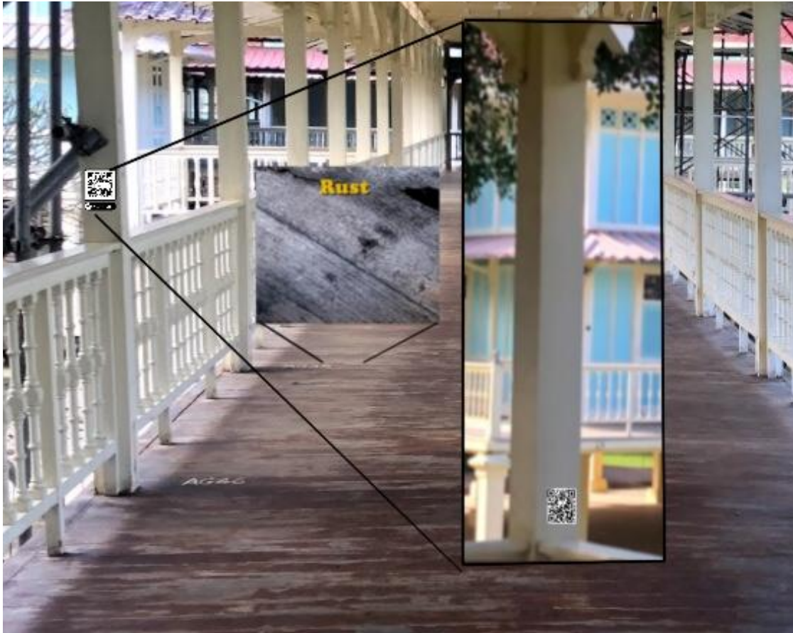
Example of implementation of QR Codes onto the pillars of the palace walkways.
