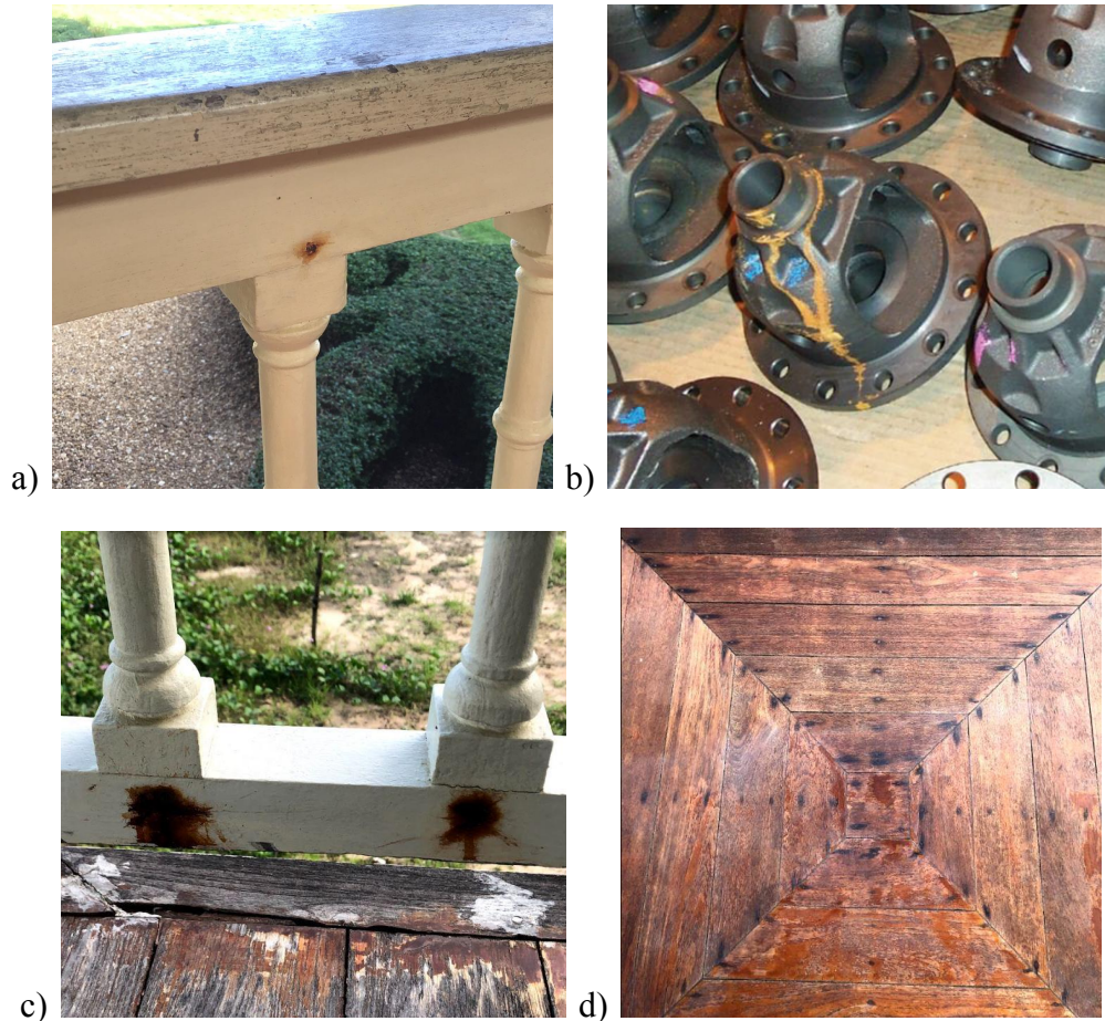
Figure 4a. Photo of red rust. Figure 4b. Formation of yellow rust on metal parts. Reprinted from Types of Rust by Armour Protective Packaging. (2019). Figure 4c. Photo of brown rust. Figure 4d. Photo of black rust.
