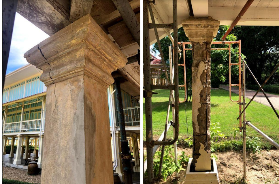
Figure 5. Photo of cracking and spalling of concrete columns around the palace area.
