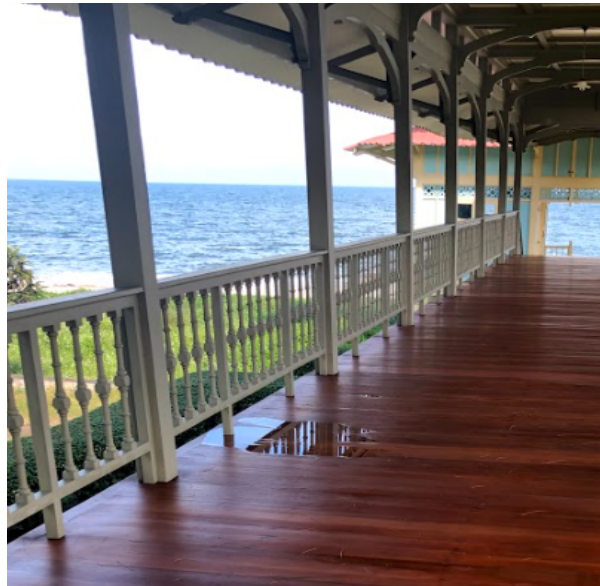
Figure 15. Photo of puddles of water on the palace floor.
