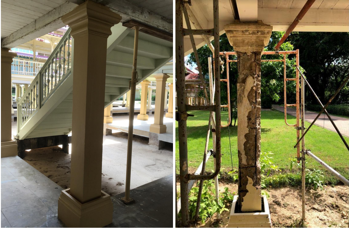
Figure 13. Photos of concrete columns without internal rebars (left) and with internal rebars that have rusted (right).
